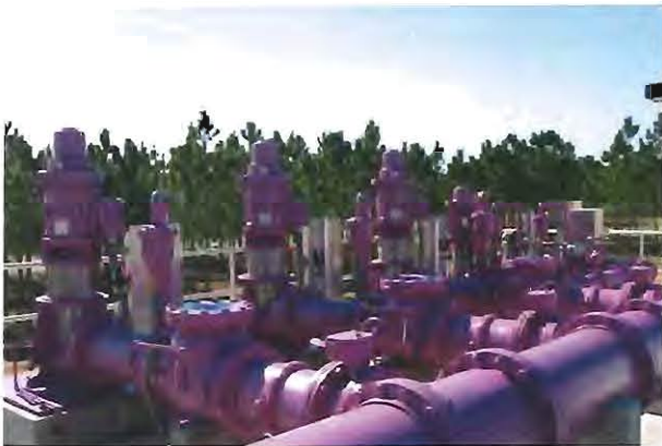
Purple pipe irrigation system
